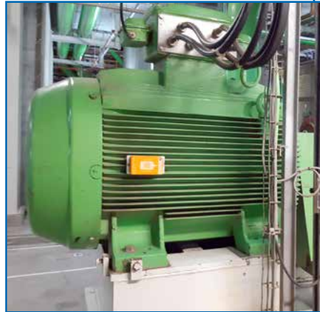
Closed Cooling Circuit Pumps PGB
