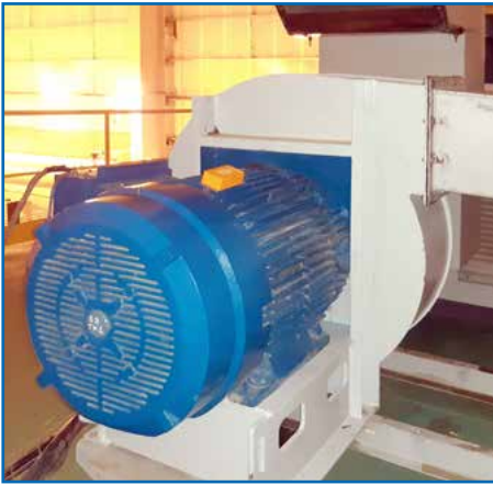
Turbine Enclosure Cooling Fans 88TK
