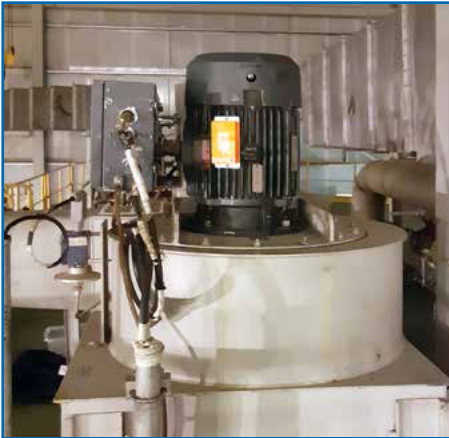
Turbine Bearing Cooling Fans 88BN
