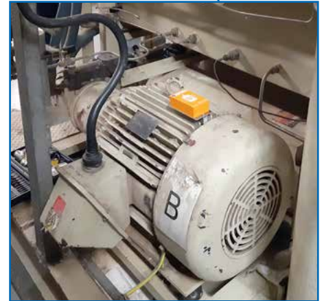
Hydraulic System Pump HPU
